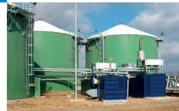
Biogas plant, Hostouň, Czech Republic
